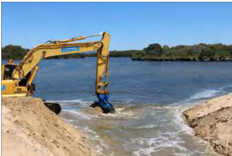
Large earth moving equipment used from time to time to open the mouth
